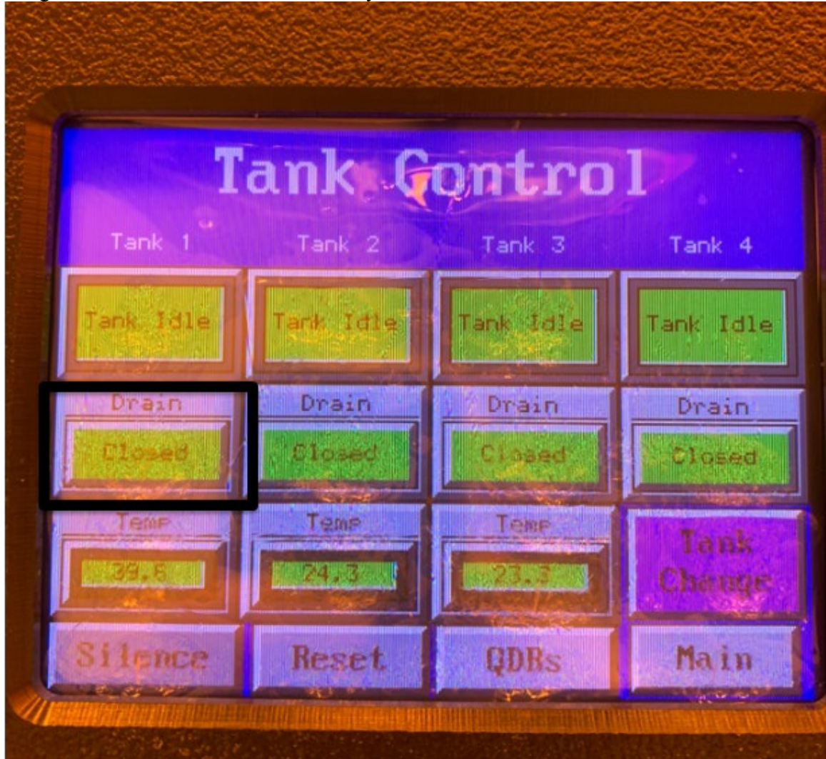
Image 2 – Drain Controls – All currently closed
