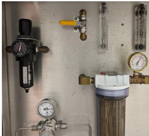
Figure 2. Air & water flow rate control panel
