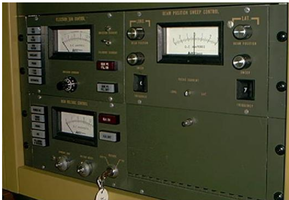
Figure 1: HVPS Controls High Voltage and Beam Control sitting on top of the CV14 power supply.
